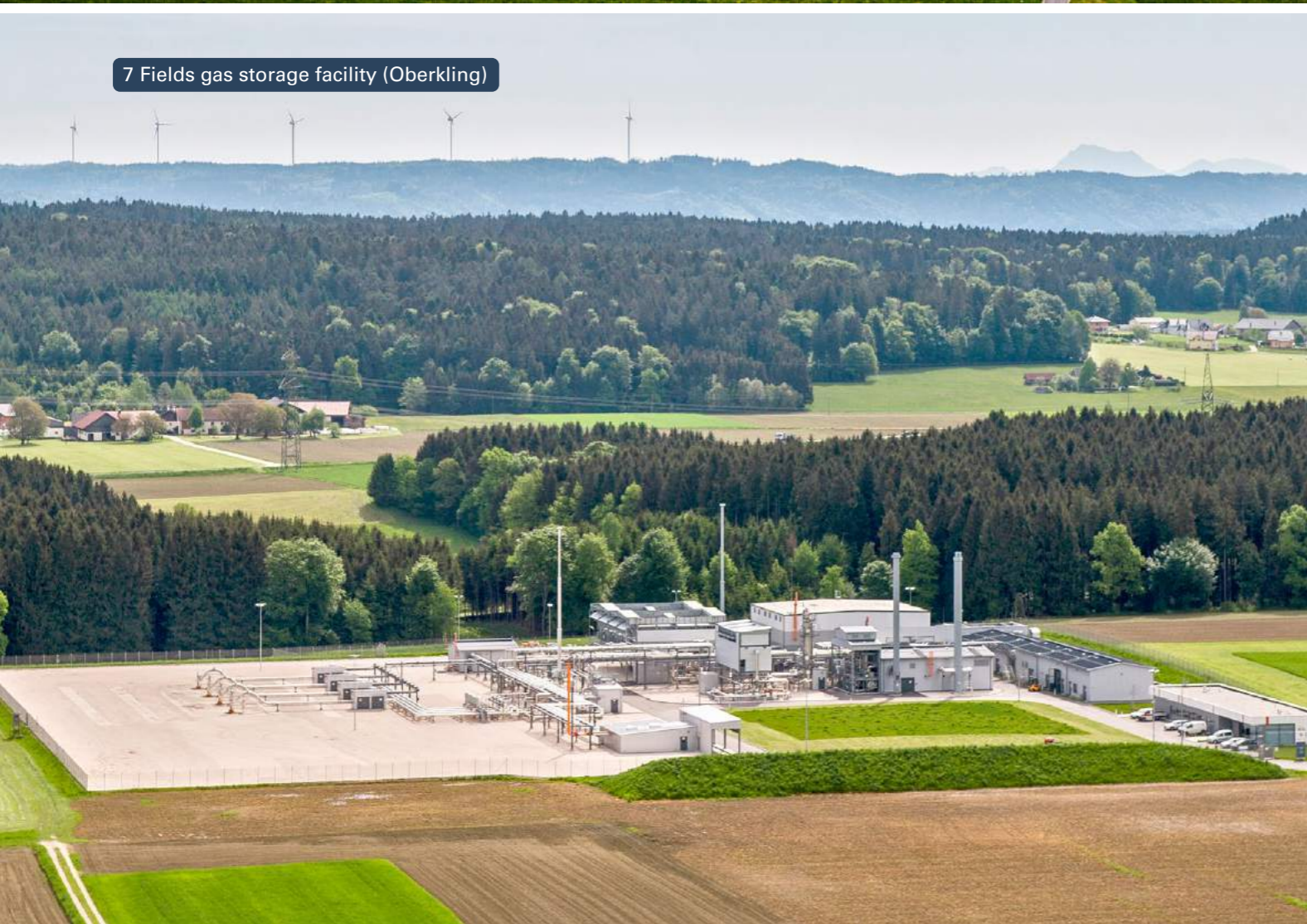
Haidach gas storage facility
